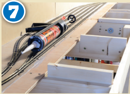
7 To ensure a strong joint between the new strip of plywood on the lower level and the original board a bead of No More Nails adhesive was applied along its length to join the boards together. Screws were then inserted to fix the new strip to the cross braces.
